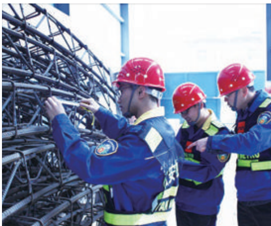
中国中铁基层进行例行安全检查 Routine safety checks by the grassroots level of CREC
