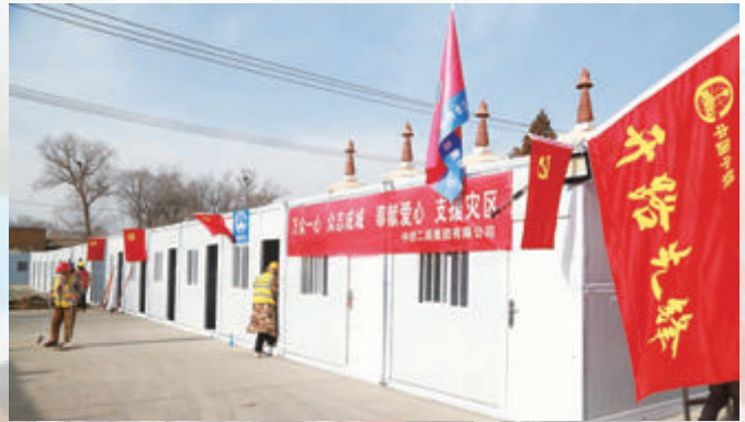
● 中国中铁全力抢建12·18积石山地震灾区临时安置房 CREC made every effort to build temporary resettlement houses in the disaster area of the 12-18 Jishishan Earthquake
