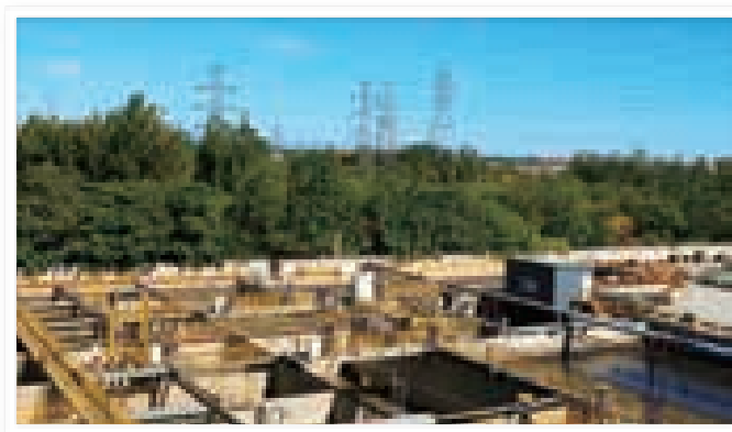
▲ “零排放、零渗漏、零污染”绿色泥水处理场地 Green cement treatment site with zero emission, leak and pollution
