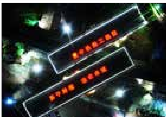
▲ 青岛新机场南进场路转体桥转体成功 Turning bridge at the south access road of new airport at Qingdao is being turned successfully
